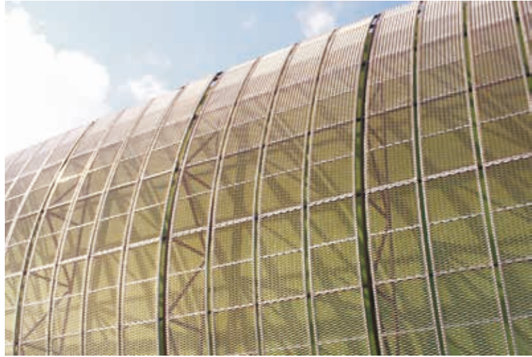
FORUM ÇAMLIK AVM / MESH CEPHE / T-T DESIGN FORUM ÇAMLIK MALL / MESH FACADE
